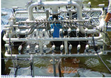
Photo 4.6 Aerators equipped in the leachate impoundment.
